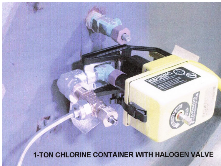
1-TON CHLORINE CONTAINER VALVES
