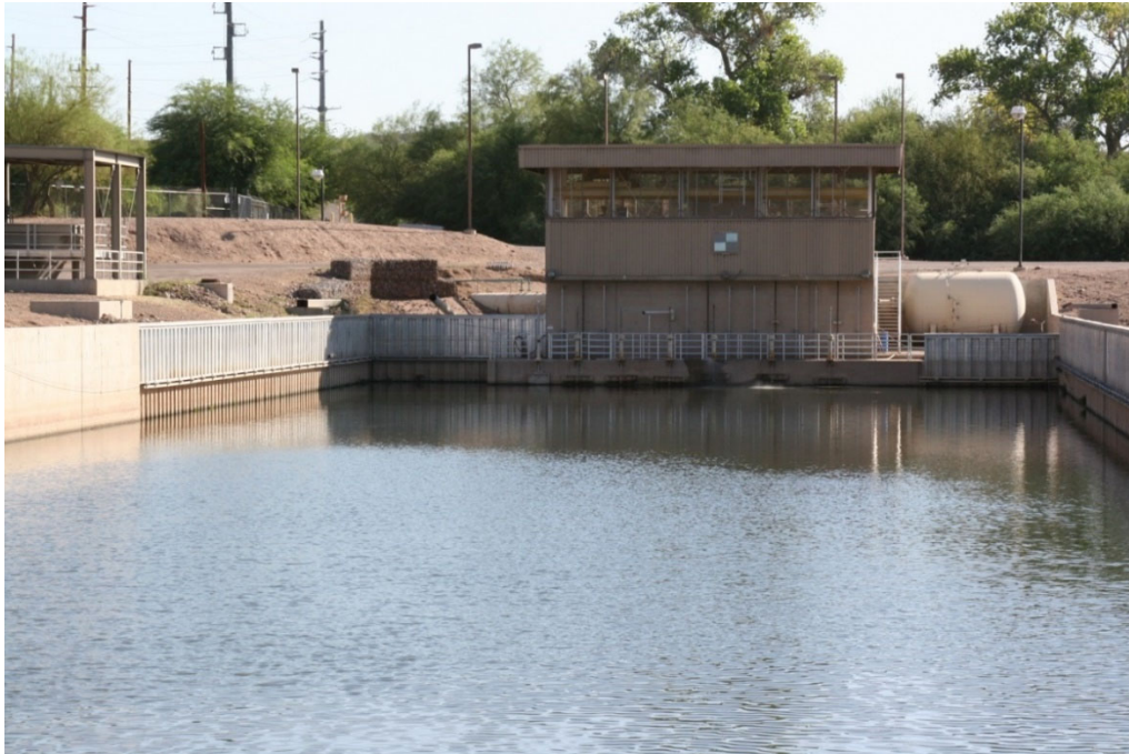
Raw Water Intake Requires corrosion protection
