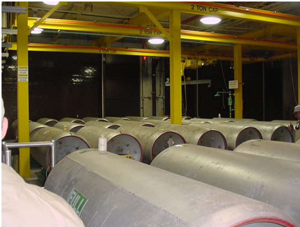
1-ton chlorine gas containers
